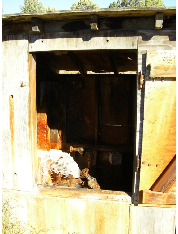
Figure 3. Pumphouse used to pump Lithia water to downtown Ashland
